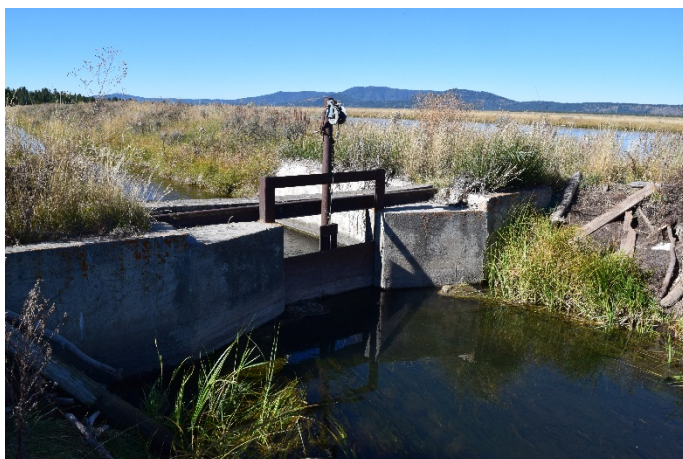
Figure 2. Headgate on Harriman Canal.
